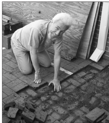
Dave Gilbert works at removing the old patio—one brick at a time.
