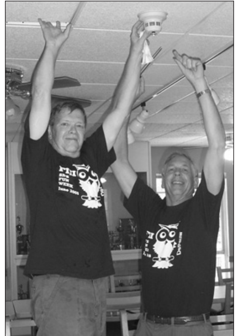
Jeff Lortz and Bud Orr work on replacing smoke detectors, lights, and fans. (Notice the special work week shirts the grads were issued.)
